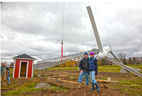
A Bergey 10-kW turbine being installed on a 120' SSL tower for a winery in Lockport, New York. Credit: Niagara Wind & Solar, Inc.
