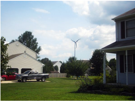
A Skystream wind turbine installation. Photo from Southwest Windpower, NREL 14935
