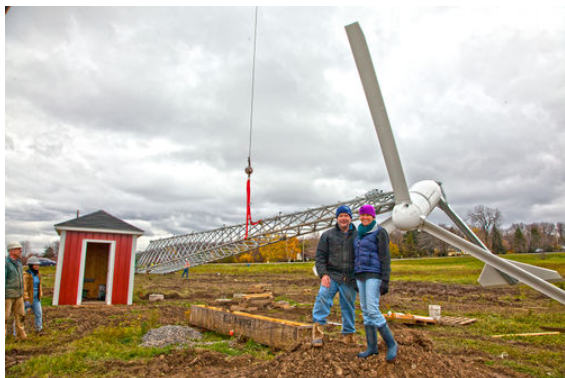
Robin and Duncan Ross installed a Bergey 10-kW turbine on a 120' SSL tower in Lockport, New York. Photo from Niagara Wind & Solar, Inc., NREL 26772
