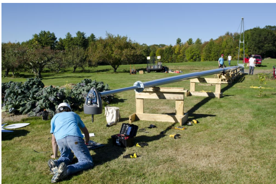
A Pika Energy small wind turbine in Gorham, Maine. Photo from Cultivate Photography Multimedia Design, NREL 30095
