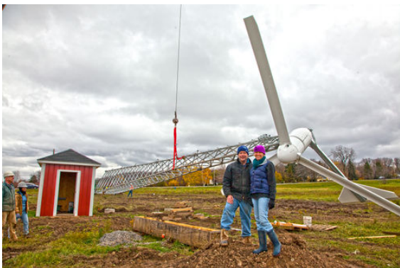
Robin and Duncan Ross installed a Bergey 10-kW turbine on a 120' SSL tower in Lockport, New York. Photo from Niagara Wind & Solar, Inc., NREL 26772
