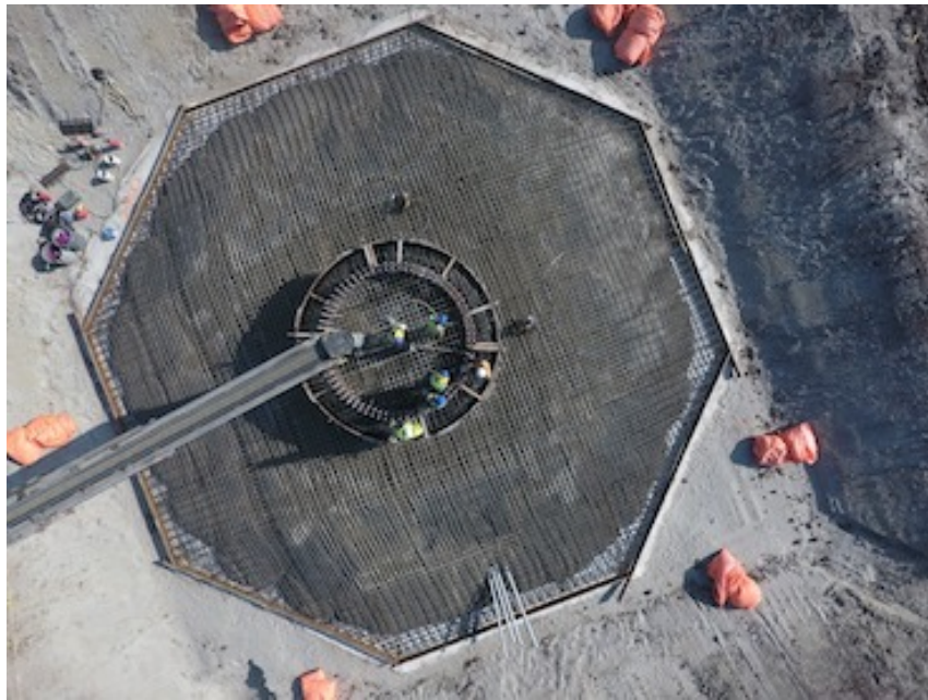
Figure 5. This foundation is part of the project infrastructure at the Amazon Wind Farm U.S. East, located in Pasquotank/Perquimans counties, North Carolina. Photo from Avangrid Renewables
